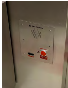
Callboxes are located inside the campus elevators. Credit: Edward Saenz
