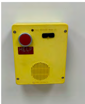
Callboxes are on all the floors of the buildings Credit: Edward Saenz
